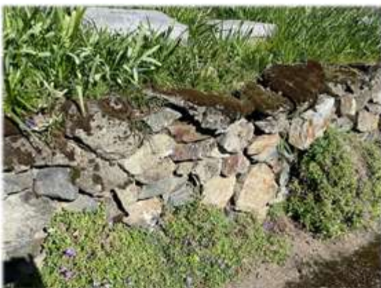
The bulging, crumbling wall
