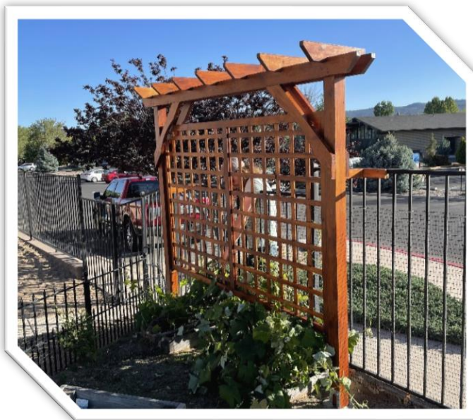
Maintaining the Preschool Grounds and building and installing an arbor in the Preschool garden made from donated materials.
