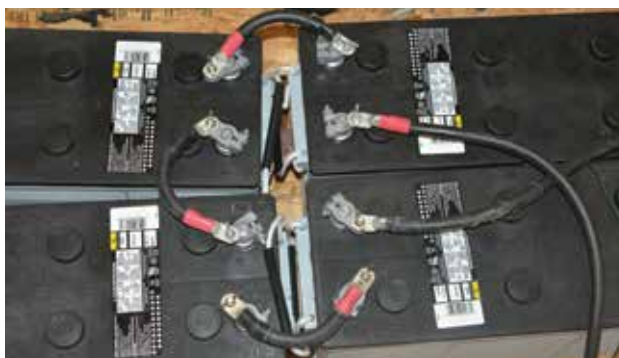
LEFT The new batteries that store the electricity sourced from the new panels on the All Saints' roof. These batteries are much smaller and more efficient than the 2007 version. RIGHT Rob Baxter in the electrical room at All Saints', on the right are the units that convert the solar energy. PHOTOS Randy Murray
